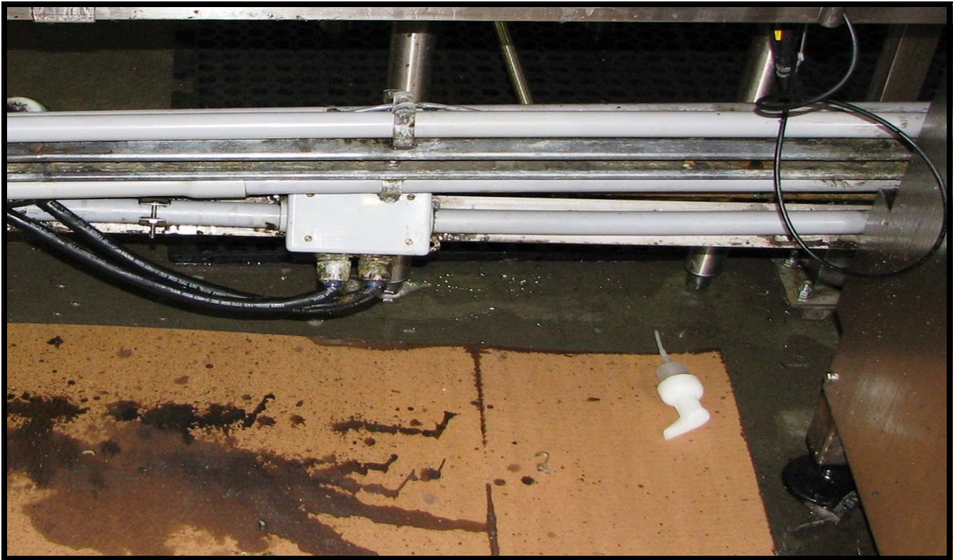
Cleaned section of conduit, wiring and framework with long lance—note the limited moisture/dirt captured on the cardboard.
